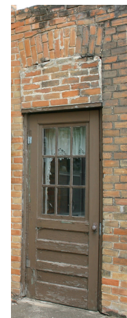
A transom window has been filled in substantially altering the appearance and functionality of this entranceway.
