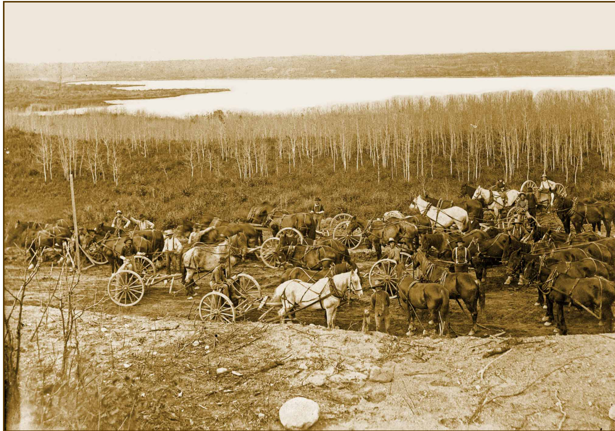
Grading the "Wakopa Branch" near the site of Neelin, with Lake Louise in the background.
