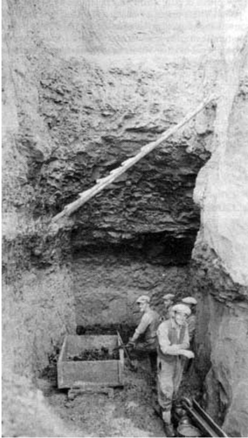
Tunnel head in the Deloraine Coal Company's ill-fated mine of the Depression years. Source: National Archives of Canada
