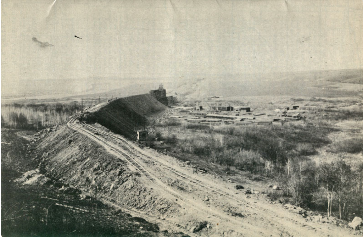
THE BIG FILL AND THE BRIDGE OVER THE SOURIS RIVER, NEAR BUNCLODY, Manitoba, about 1905. The two tracks on the fill allowed the train of loaded dump-cars to proceed to the dumping position, while the empties returned on the other track to be refilled. Photo Gilford Copeland
