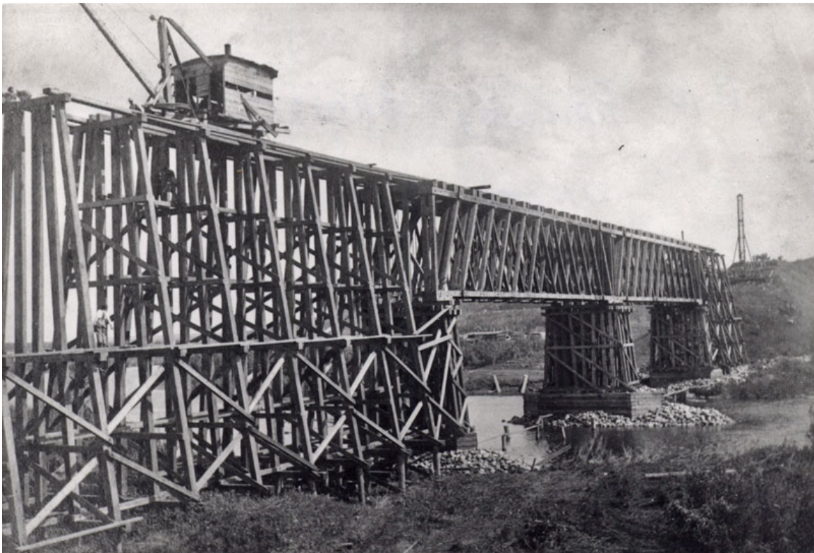
BUILDING THE SINGLE-TRACK, TWO-SPAN, BOX-GIRDER, WOODEN BRIDGE OVER the Souris River near Bunclody, Manitoba, on June 19, 1906. Photo Gilford Copeland
