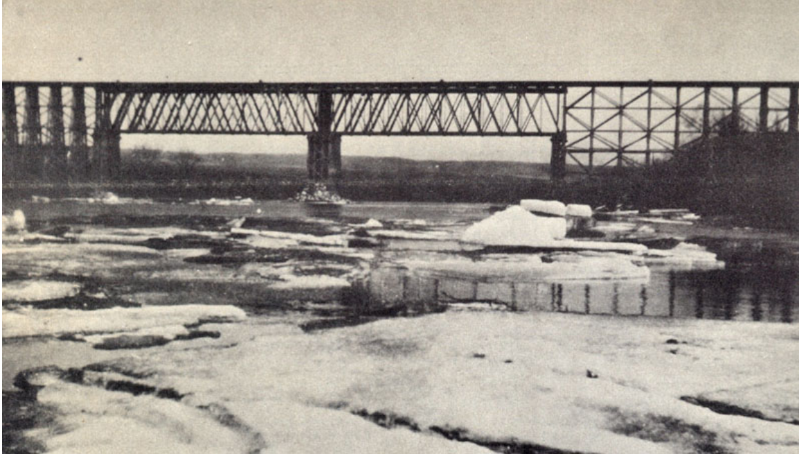
BS&HB'S WOODEN BRIDGE OVER THE SOURIS RIVER WAS REBUILT TO A steel box-girder structure in 1929-30. The spring run-off remained substantially the same and the ice-cakes battered the central pier each spring. Photo Gilford Copeland
