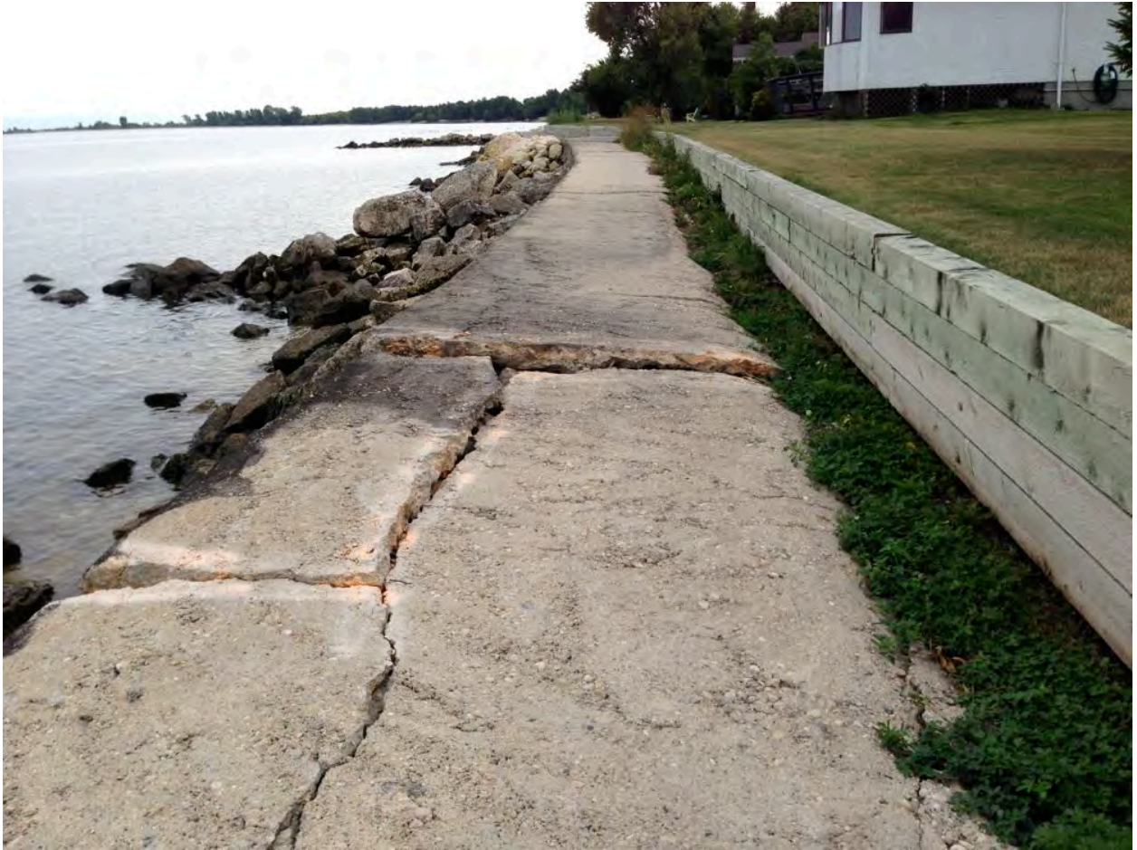
Major cracks developed in 2013 making it treacherous for cyclists and pedestrians alike (photo E Ward.)
