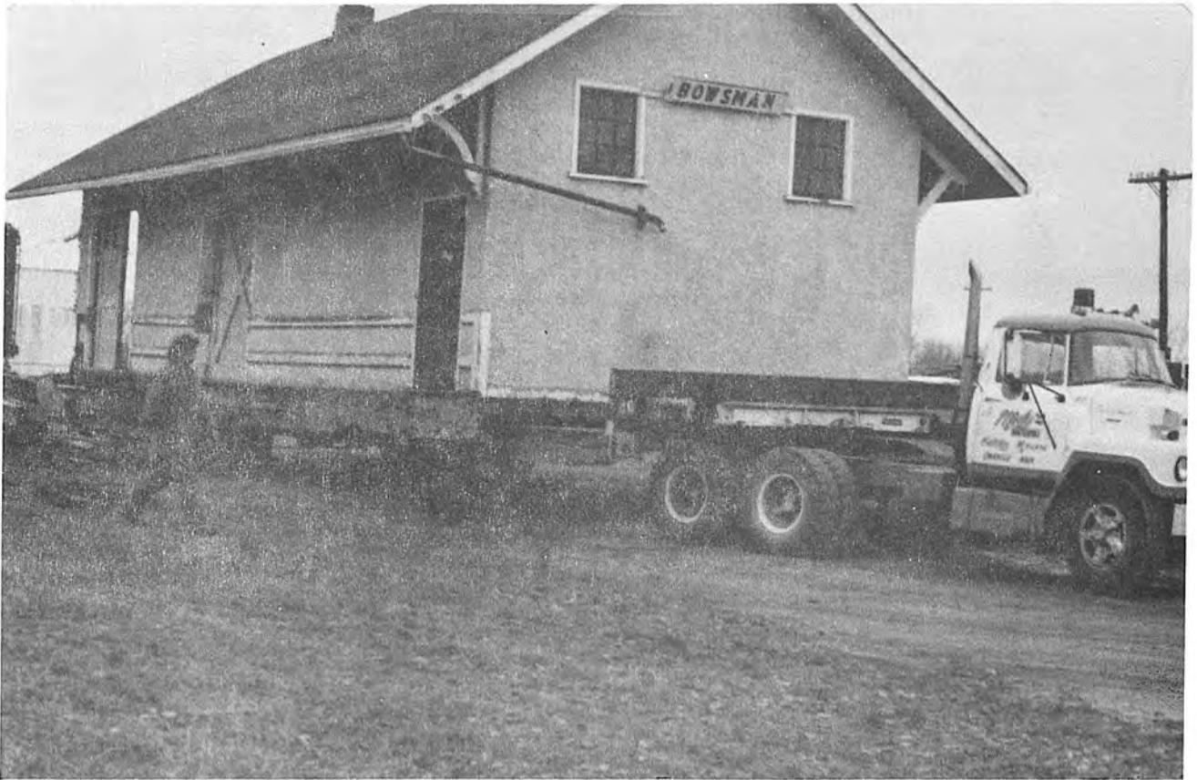
The warehouse of the station had to be detached from the main building to facilitate the move.
