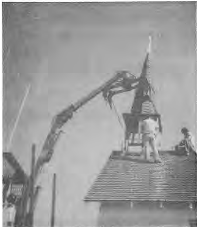
Using a cherry picker on loan from a local contractor to replace the steeple on a church.
