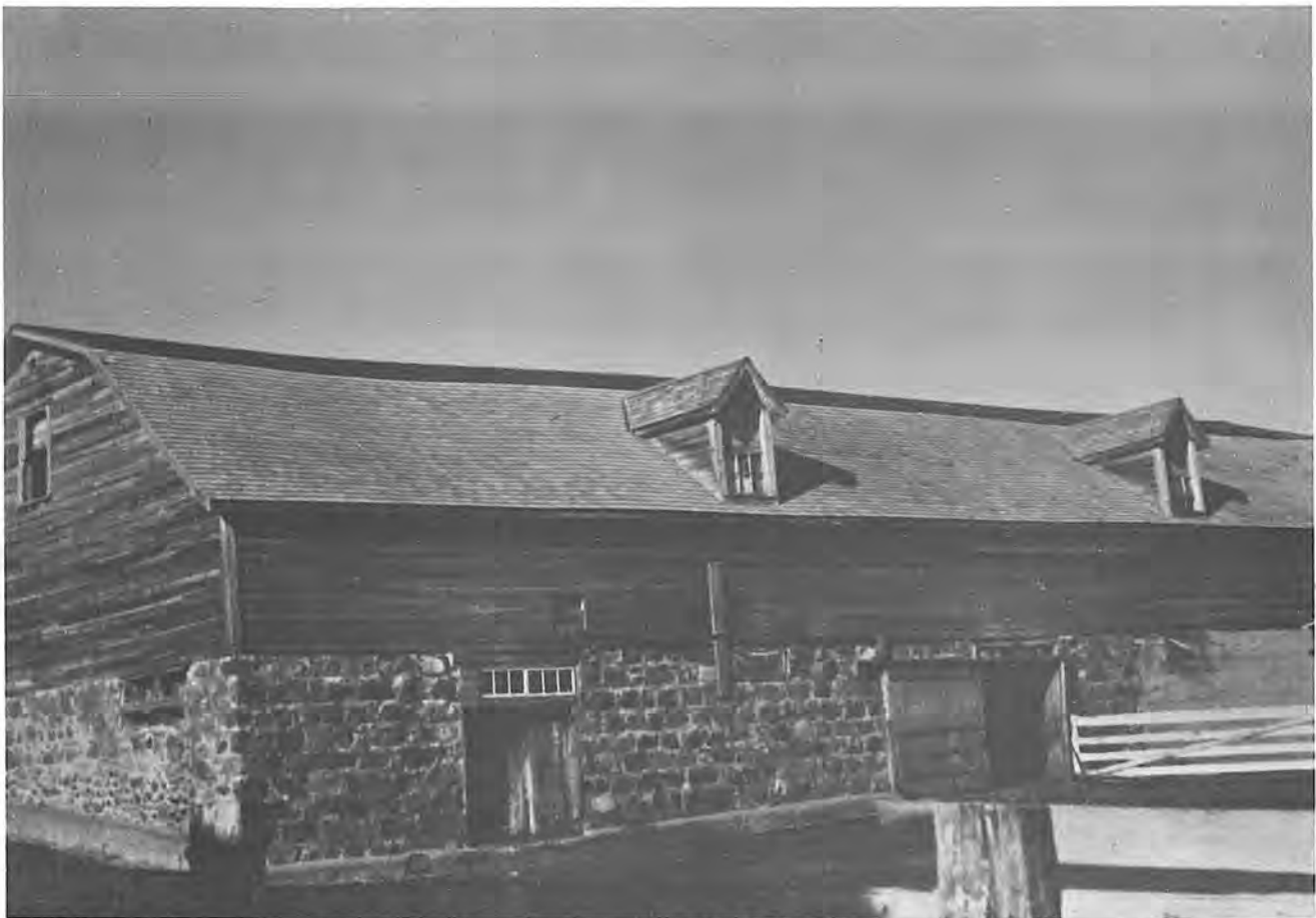
A 'Bank' barn, of fieldstone, built in 1898, frame construction added in 1907, Virden
