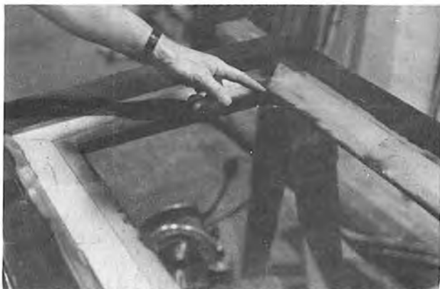
Firedamage to the rear of some of the panels
