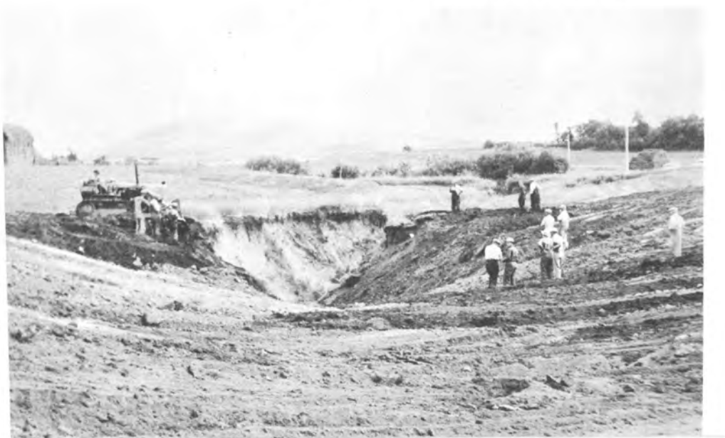
51. Gully-filling in progress - when completed, was seeded down to grass with a nurse crop of winter rye
